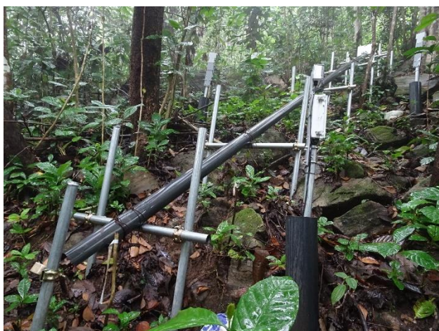
Figure: Slope displacement monitoring equipment
